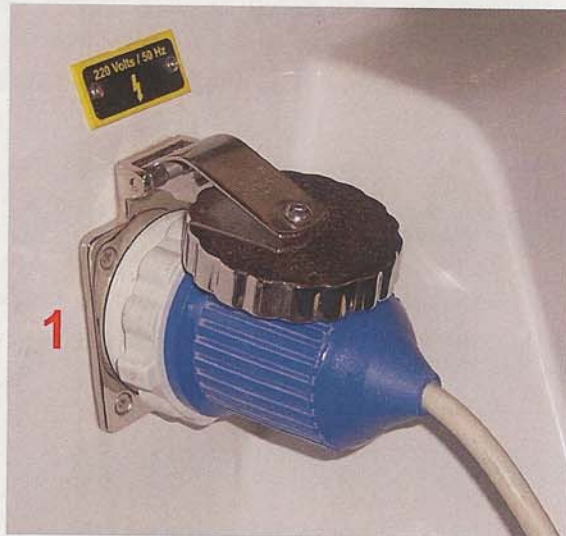
Shore power socket
