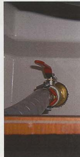
Engine water valve: Thru-hull fitting with valve
