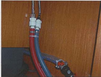
Kitchen tap connection
