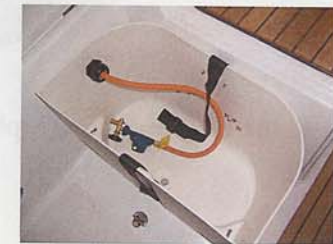
Gas cylinder locker
