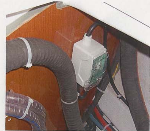
Access to the circuit breaker through the starboard aft locker under tiller seating
